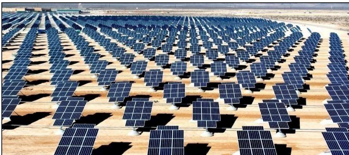
Fig. (II.22) Photo illustrant un champ photovoltaïque
