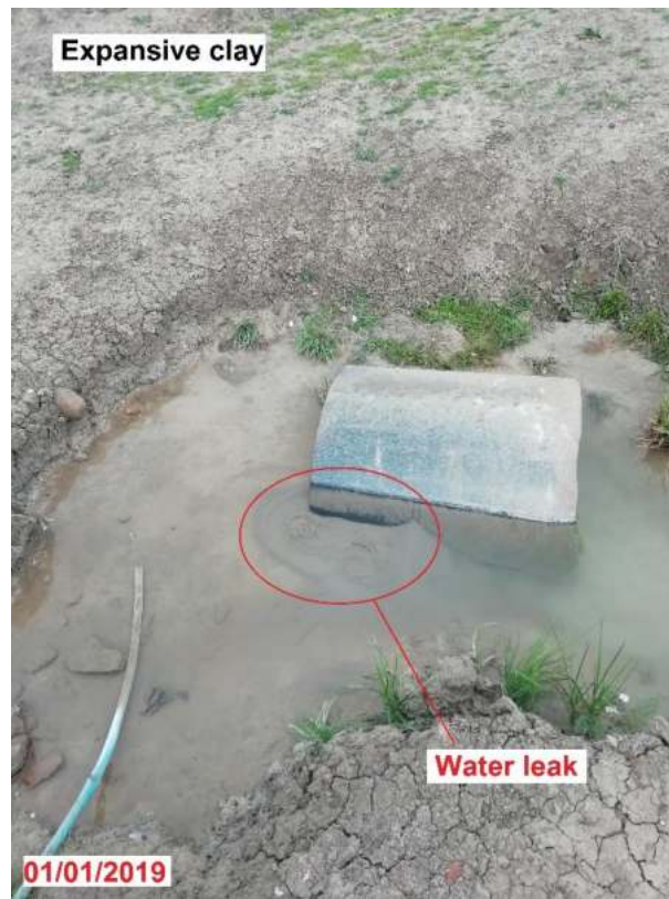
Figure 3-6 Water leakage point at Aine-Tine site
