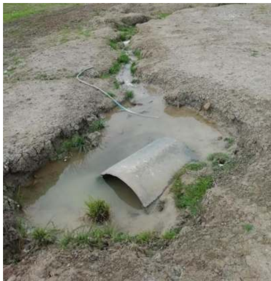
Figure -4. Water leakage point recorded at the Aine-Tine slope
